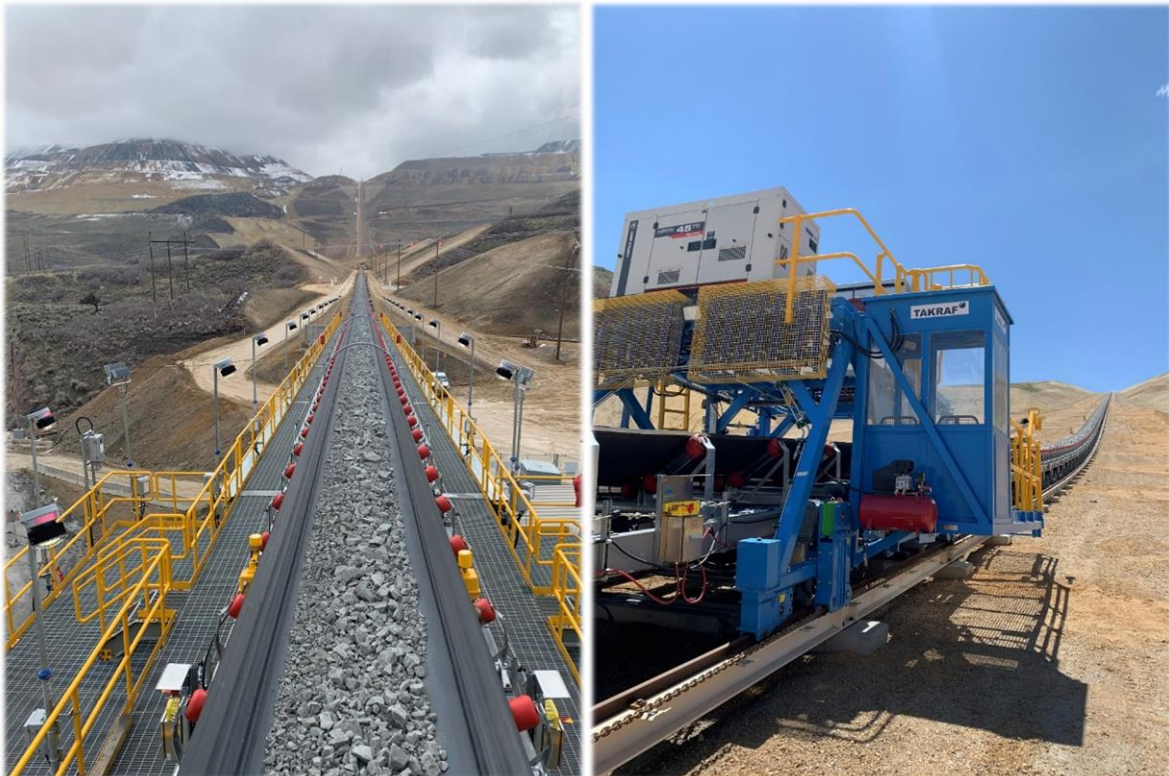
TAKRAF's US relocation project showing new downhill conveyor managing a 15 degree slope carrying ore to processing facilities on the left and TAKRAF maintenance cart for safe and efficient idler maintenance in position on the right.
